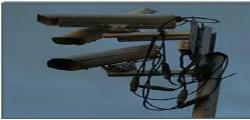
Fig. 1 Example of CCTV camera
