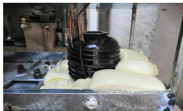
Figure: Heat Exchanger tank with puff.
