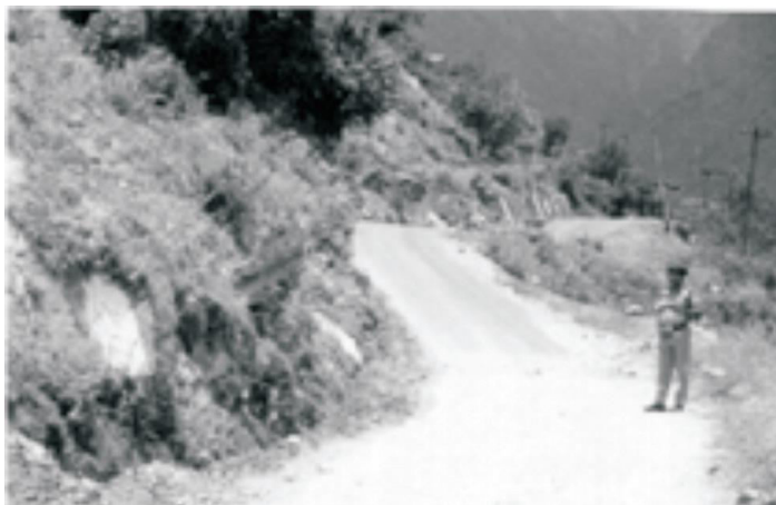
Fig 2.9 Condition of road stretch after Monsoon Rains
