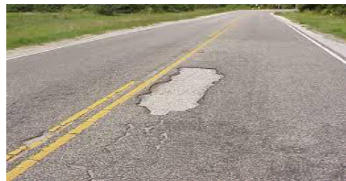
Figure 1.3: Surface Layer Delamination
