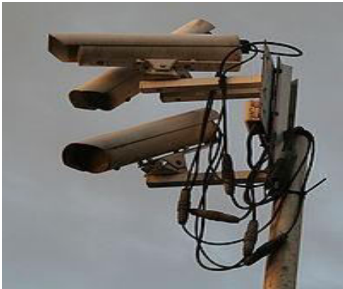
Fig 1.1: Closed-circuit television (CCTV)
