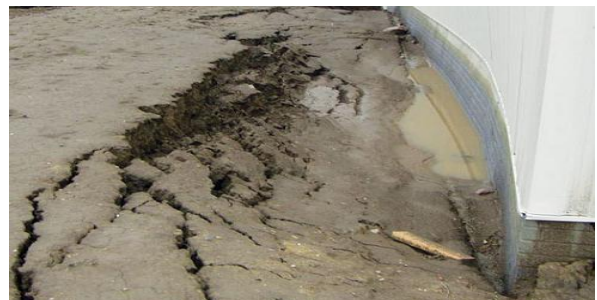
Figure:1 Damages due to shrinkage
