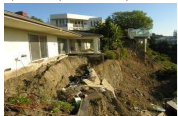
Figure: 2 Damages in structures
